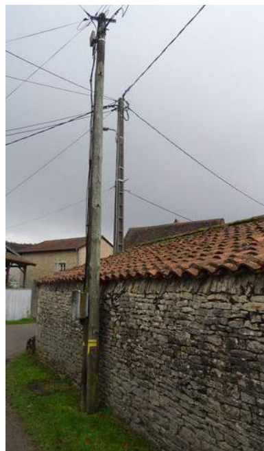
Poteaux ciment Sagy-le-bas
